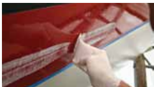
Fill along boottop
